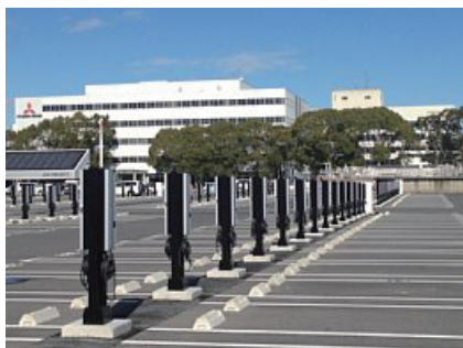
Fig. 9 Normal chargers for employees (Mitsubishi Motors Okazaki Plant Employee Parking Area) (56)
